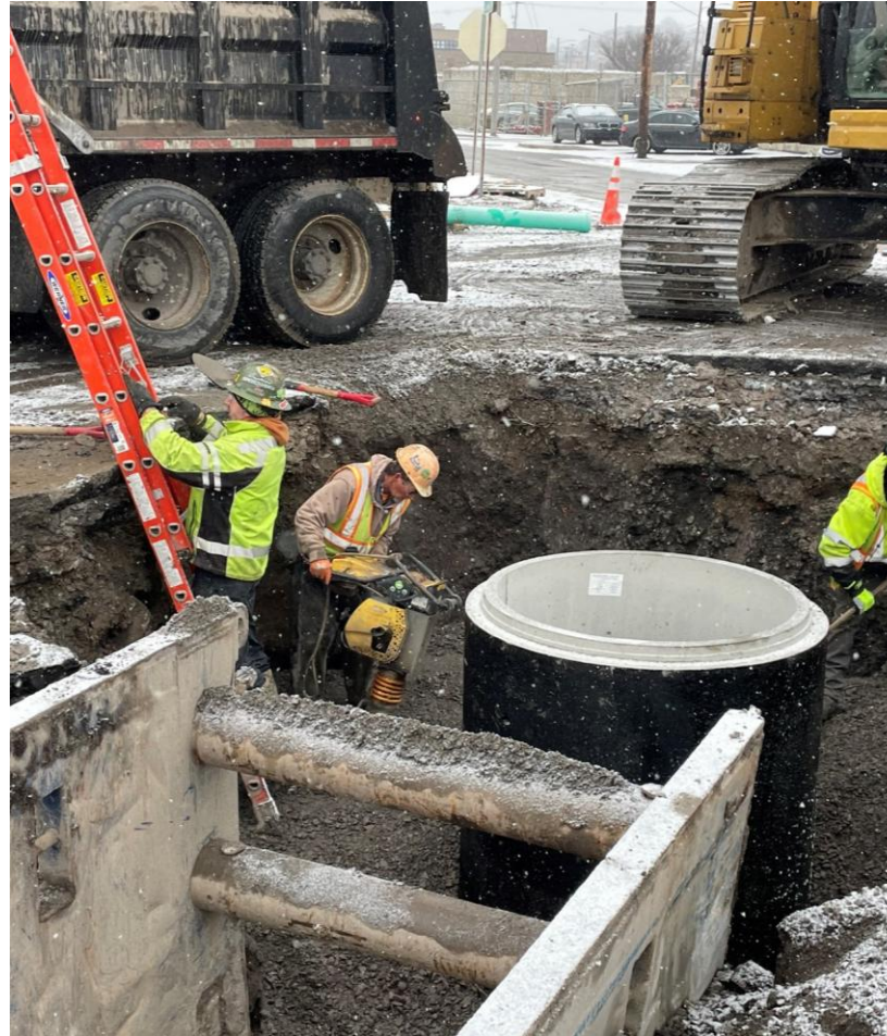
New Stormwater Trunkline
